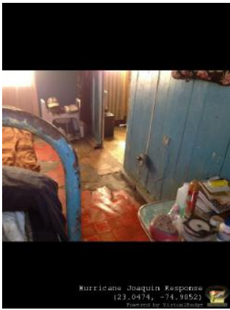
Water Damage in Home 23.0474, -74.9052
