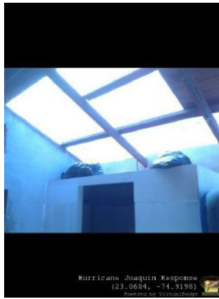
Major Roof Damage 23.0604, -74.9198
