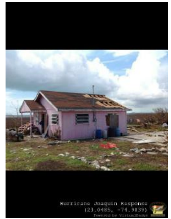
Major Roof Damage 23.0485, -74.9039
