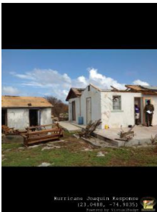
Partially Destroyed Home 23.0488, -74.9035
