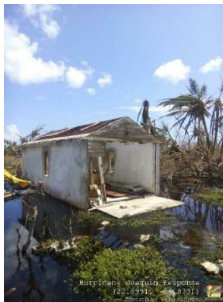
Partially Destroyed Home 22.8991, -74.8731
