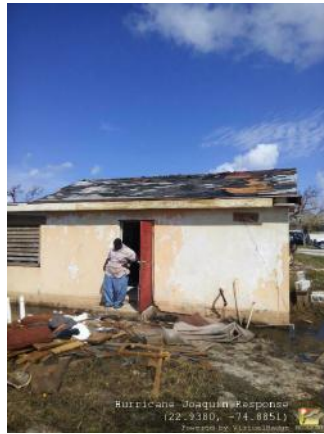
Major Roof Damage 22.9380, -74.8851
