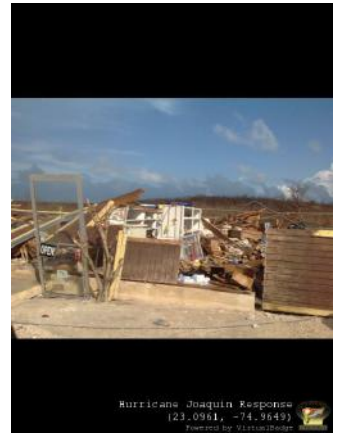
Partially Destroyed Home 23.0961, -74.9649
