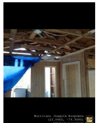
Major Ceiling Damage 23.0460, -74.9046
