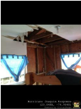
Wall and Ceiling Damage 23.0481, -74.9048
