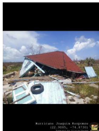
Completely Destroyed Home 22.9005, -74.8730
