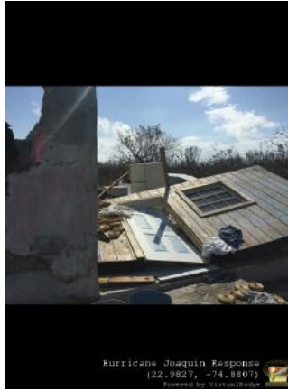
Completely Destroyed Home 22.9827, -74.8807
