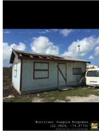
Major Roof Damage 22.9824, -74.8770
