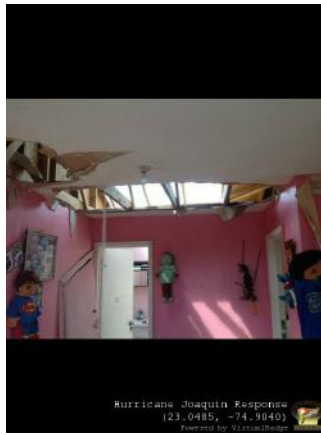
Major Roof Damage 23.0485, -74.9040
