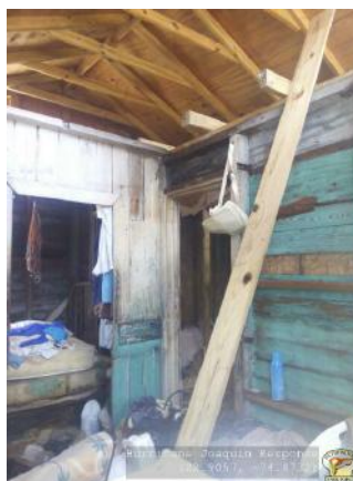
Major Ceiling Damage 22.9057, -74.8732
