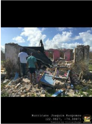
Completely Destroyed Home 22.9827, -74.8807
