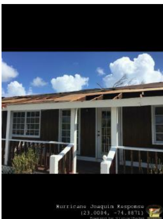
Major Roof Damage 23.0004, -74.8871
