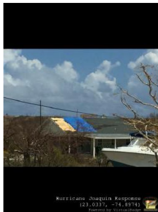
Major Roof Damage 23.0337, -74.8974
