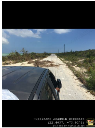
Debris on Road
